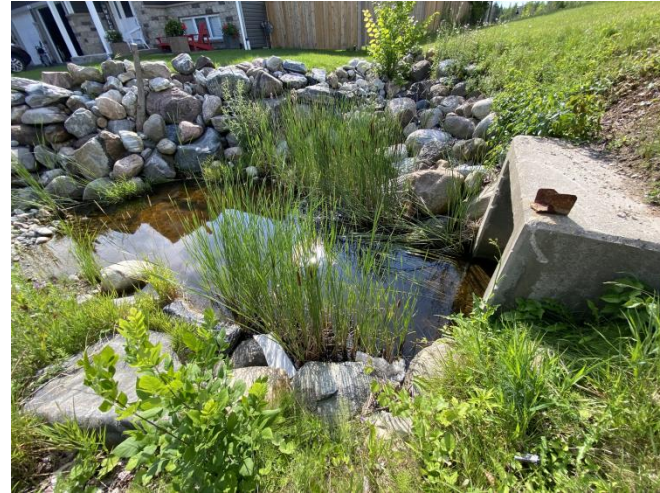
Photograph 2: Outlet pool on downstream (north) side of Beachwood Road culvert – direct fish habitat
