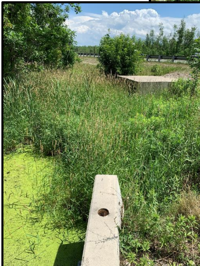
Photo 10 (left): Bayshore Creek enters the property through box culverts on the north side of Highway 26. The area around the culverts holds water into the summer, but there is no standing water on the property (July 29, 2021).
