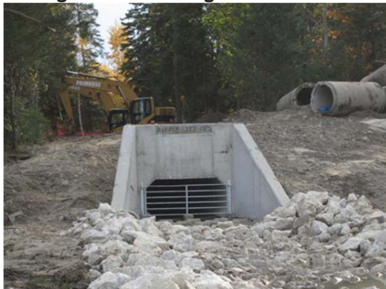
Figure 9: Existing 67 th Street Outlet
