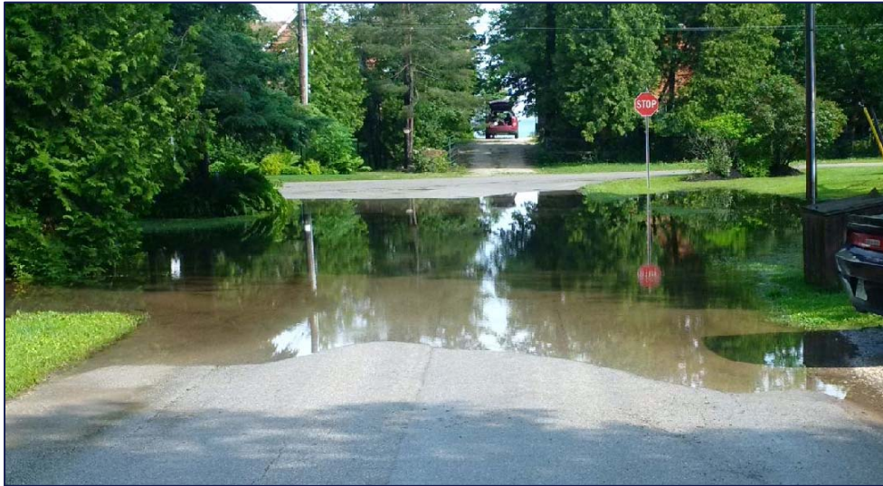
Figure 11: Flooding at 63 rd Street North and Shore Lane
