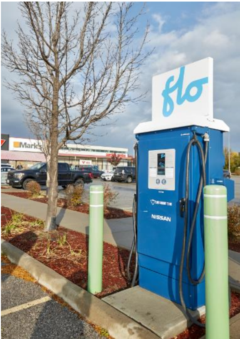
Figure 39: Smart DC - 50 kW Level 3 FLO charger
