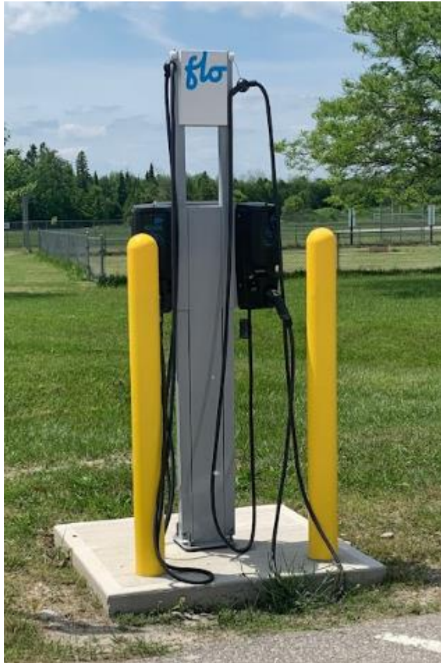
Figure 38: Level 2 - CoRe+ chargers + pedestal + bollards
